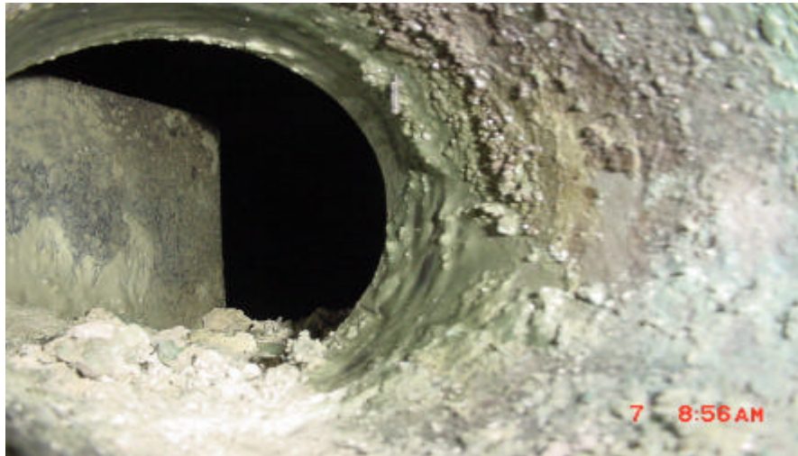
Figure 5 Acid Formation in Piping
