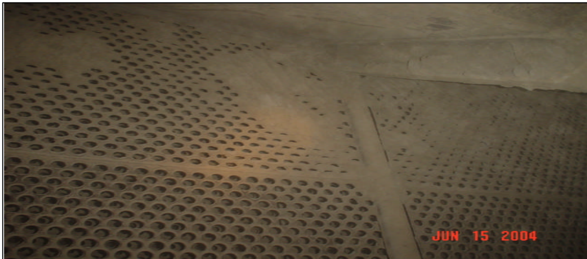
Figure 3 Blocked Distribution Plates
