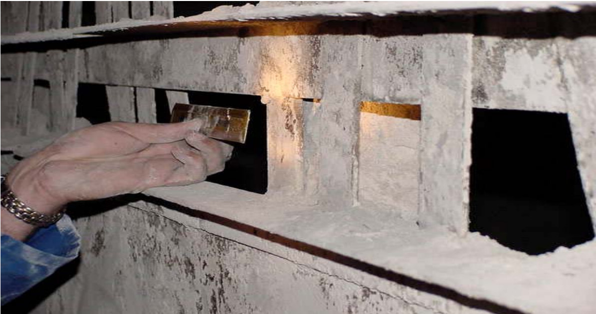
Figure 2 Previously blocked outlet distribution screen
