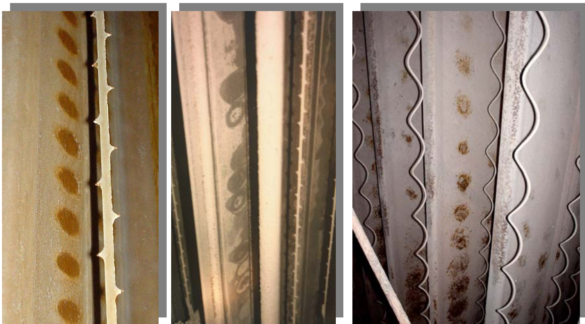
Photo 1: Details of poor current discharge coverage on collector electrode plates
